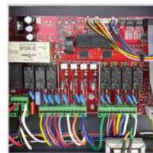
Centralizing main PCB
